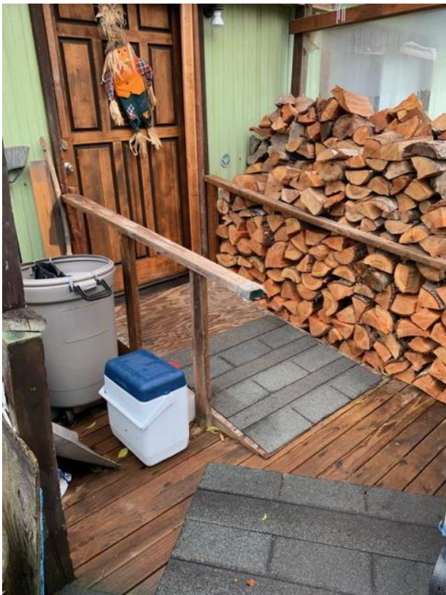
Old dangerous ramp
